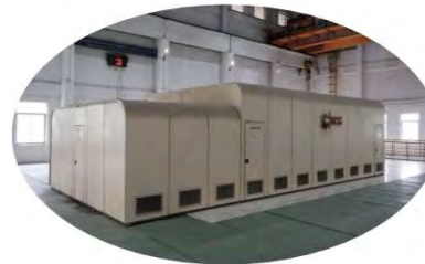
Waste heat generator
