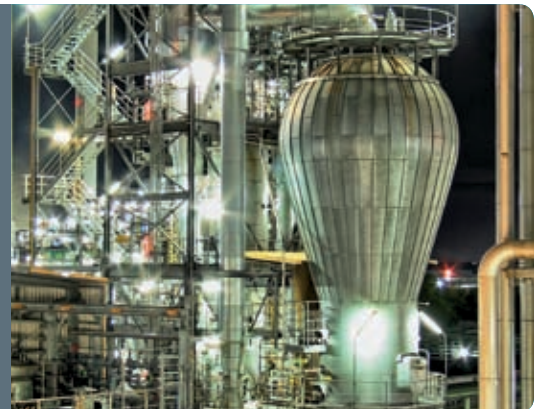
Spherilene process plant – LyondellBasell, Wesseling, Germany
