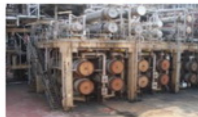
Shell &amp; Tube Heat Exchanger
