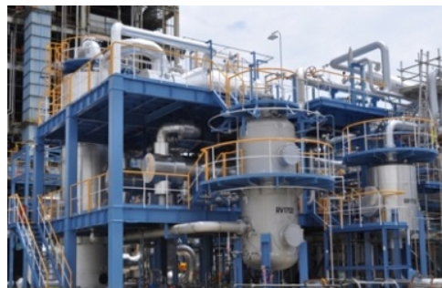
Expanded portion of the gasification facility
